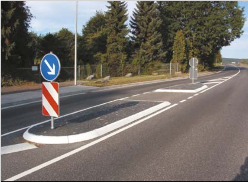
K 106 by-road, Neuwied-Niederbieber: Kerb of a traffic island stuck to the asphalt with SILIKAL® Mortar R 17
